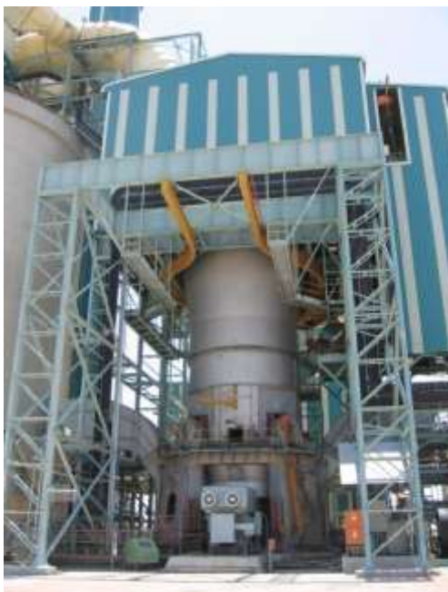
Figure 5. first VRM installed in Hard Rock Application (BWI 25 kWh/t) for grinding phosphate Rock at Foskor RSA
