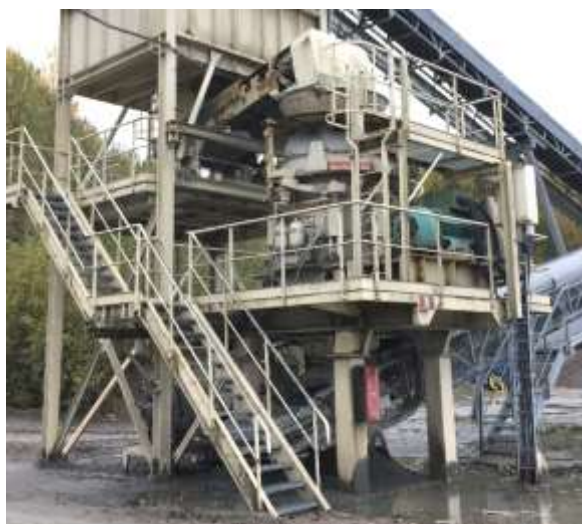
Figure 3. The CCU is installed on a Metso Nordberg HP4.
