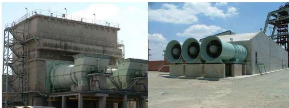
Figure 2. A vertical fill-packed tower BAC and multi-stage horizontal spray chamber BAC (Greth, 2018) Source: Roman et. al, 2013)
