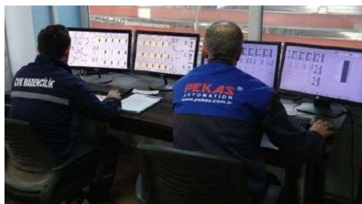
Figure 8. Process Control Room of a Lead & Zinc Plant Designed and Built Locally (Courtesy of Pekas)
