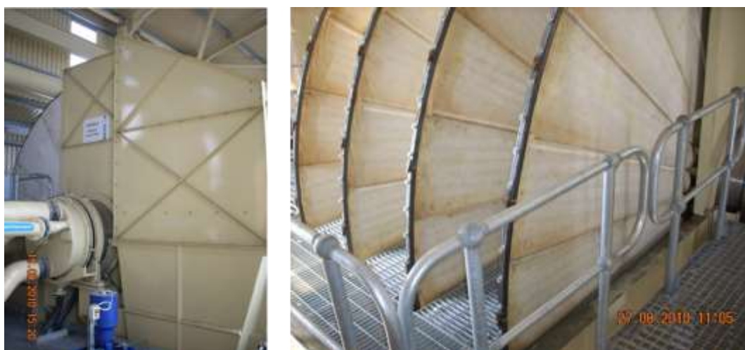
Figure 3. Disc filter (176 m 2 filter area) assembled in the gold/copper mine; view of control head side (left); and view of the four filter discs with walkways (right)
